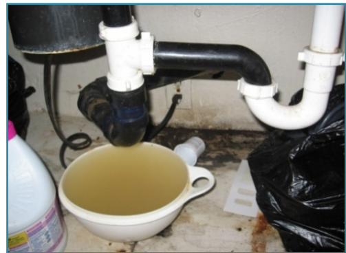
Water leaks from pipes and faucets were a major structural problem in most homes.
