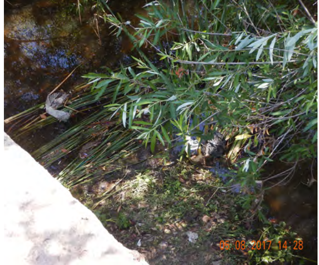
Photo 4 – Closer inspection of MS4 outfall, which collects three separate drainages from north. This field trip took place two days after a significant rain event; note the brush flattened from storm water rushing from outfall, thus, pushing trash farther down the creek.
